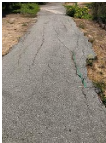
Asphalt Trail in Poor Condition
