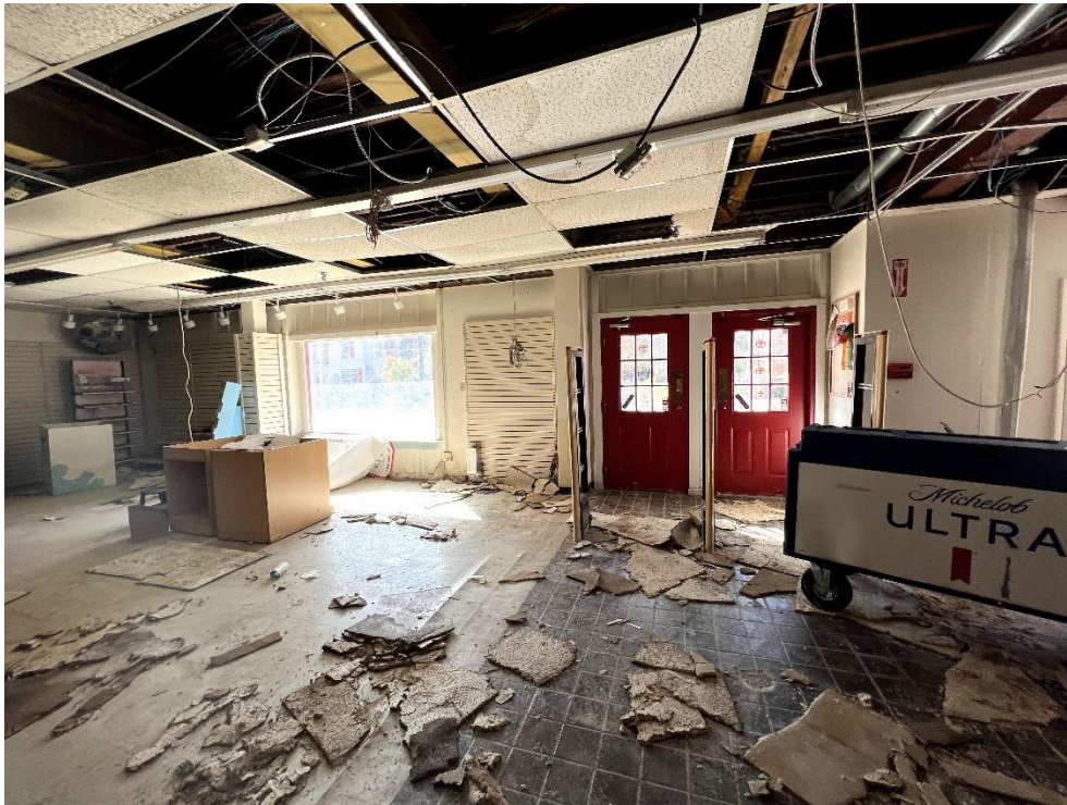
View of First Floor south façade wall, vinyl and ceramic tile flooring, drop ceiling, camera direction south
