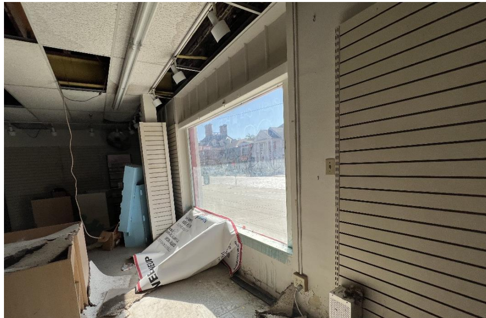
View of First Floor picture window, gypsum and slat wall materials, camera direction southeast
